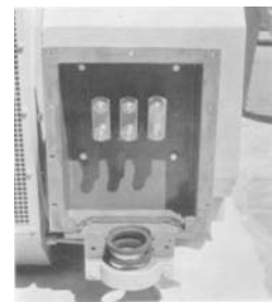
Fig. 8. View of the rotor terminal box
